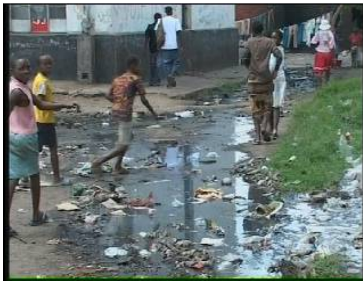
Burst sewer pipes in a high density suburb in Harare © F Machingura/TARSC 2008
